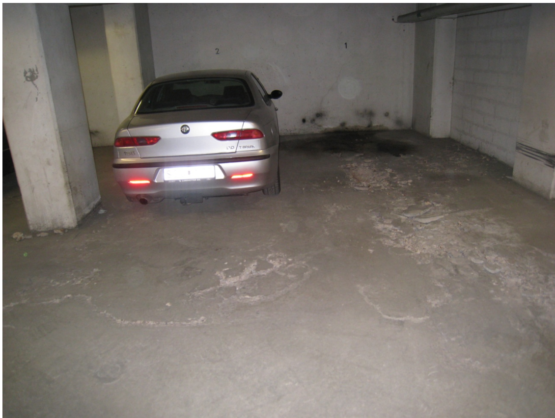
Figur 2. Betongskador i garage
