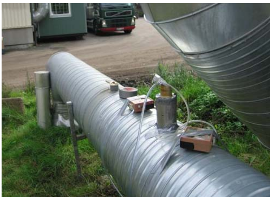
Figure 10: Picture of sampling in the pipe before the biofilter
